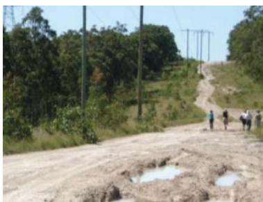
Plate 3.1 Eroded Access Tracks along Powerline Easement
